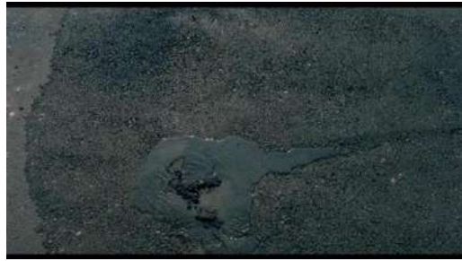
Figure 5.19 Holes that seeped water
